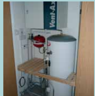
A mechanical ventilation with heat recovery unit above the hot water cylinder
