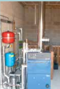
The biomass boiler for the Code Levels 5 and 6 houses
