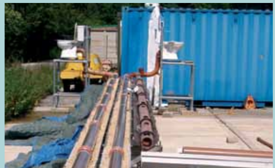
The drainage test rig
