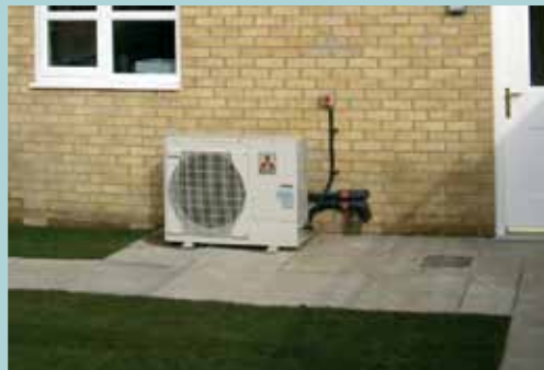
The air source heat pump of the Code Level 3 house
