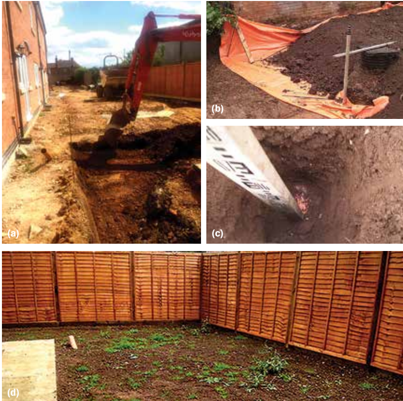
Figure 6.10 Remediation on a small site, excavating soils (a), laying membrane and topsoil (b), verifying the depth of topsoil (c) completed remediation, before laying turf (d)
