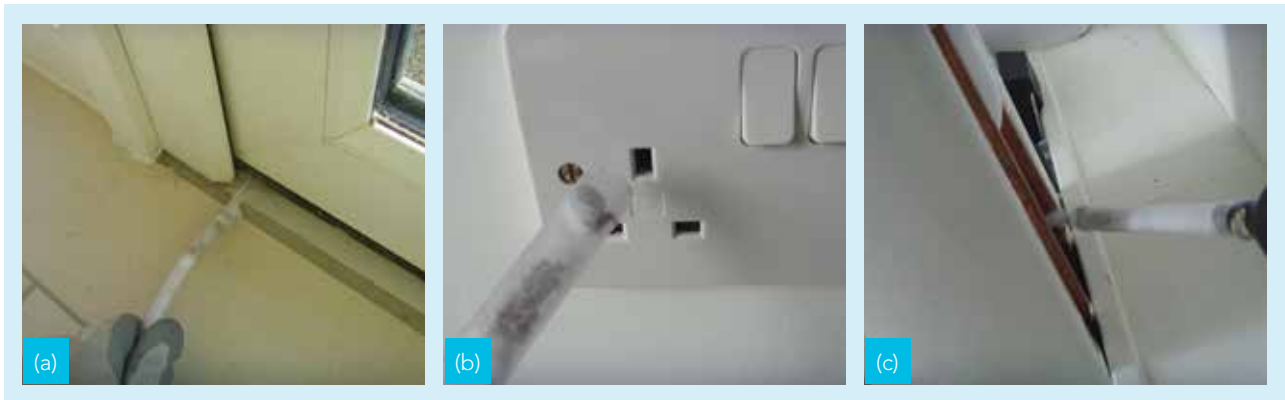
Figure 6 Typical air leakage paths in Greenwatt Way homes (a) under back door (b) through wall sockets (c) through gap behind bathroom basin
