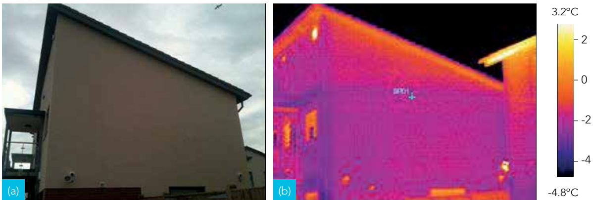
Figure 9 (a) West façade of Home 5, (b) corresponding thermal image shows some heat loss at eaves level
