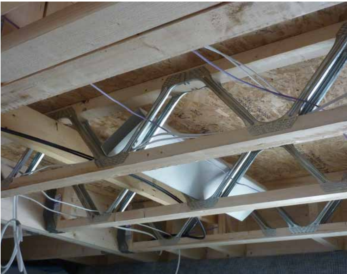
Figure 12 Flat ductwork (as specified) clashing with joist webs
