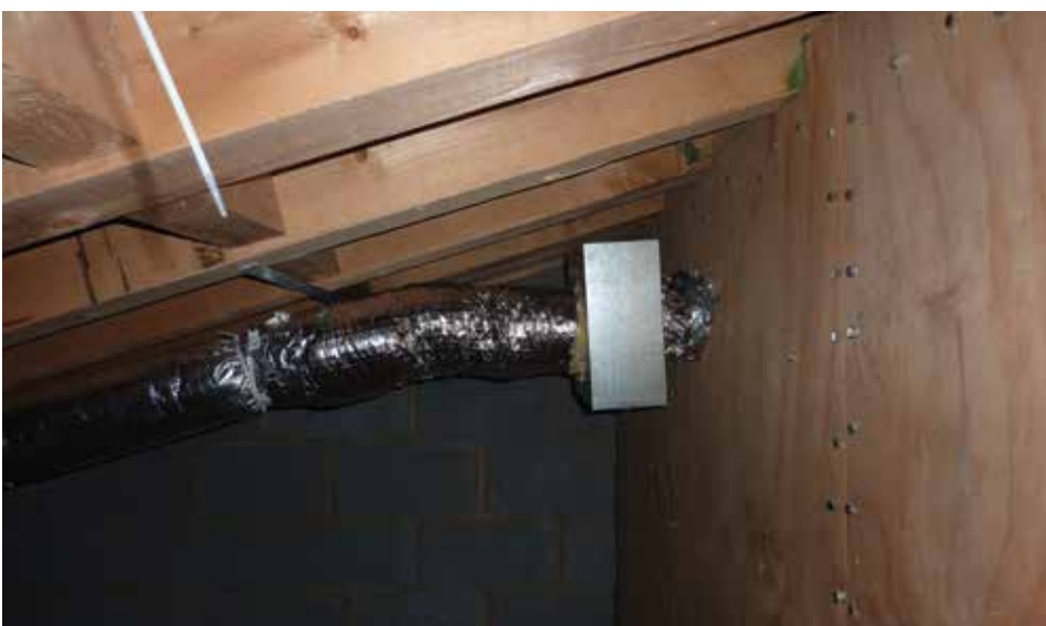
Figure 23 Filter box installed in supply air duct inside loft
