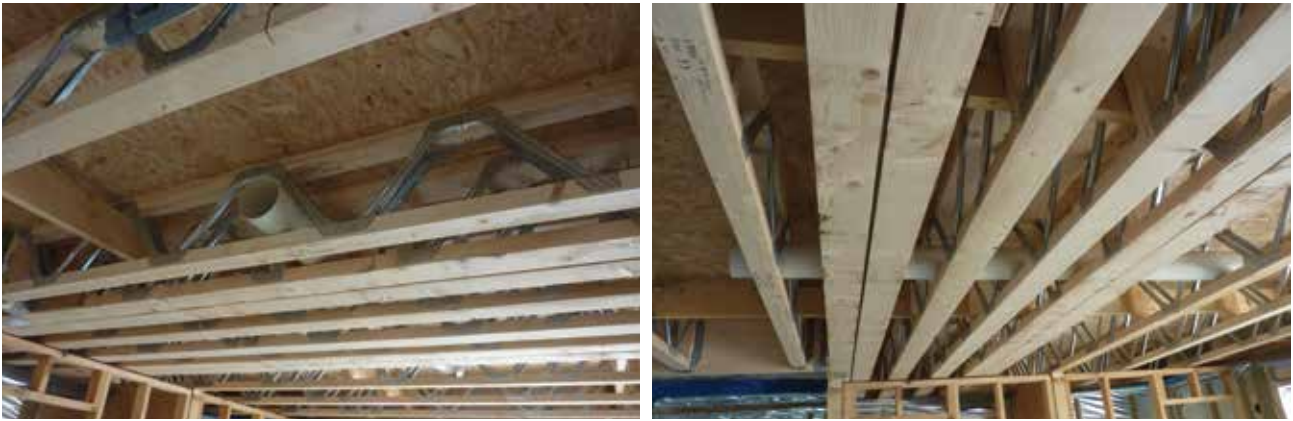
Figure 13 Round ductwork allowed direct runs from risers to air valves and could be installed in long lengths, minimising the number of connections
