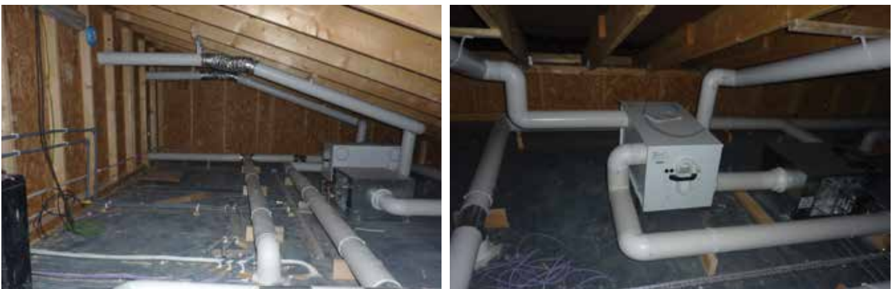
Figure 14 MVHR fan unit and associated distribution ductwork in the loft
