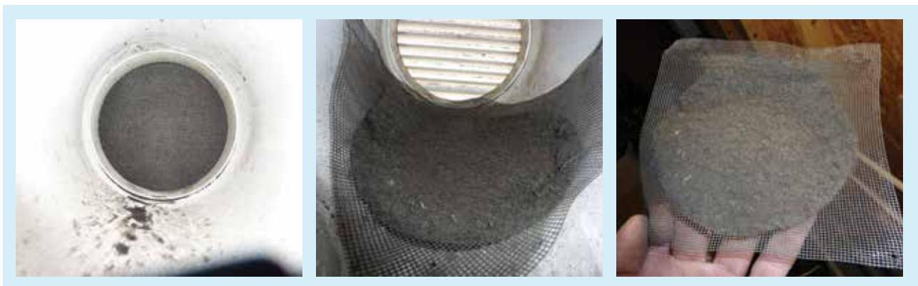
Figure 22 Fly screen removed from a supply air valve – almost totally blocked by build-up of debris
