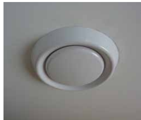
Figure 17 Supply and extract valve commissioned to near shut
