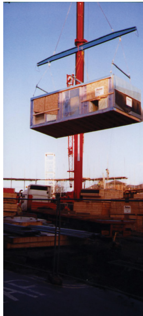
Figure 13 The modules were craned into position after the erection of the steel staircases and walkways
