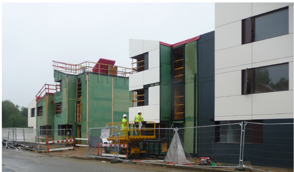
Figure 26 The latest homes under construction. The timber superstructure and roof are assembled without scaffolding
