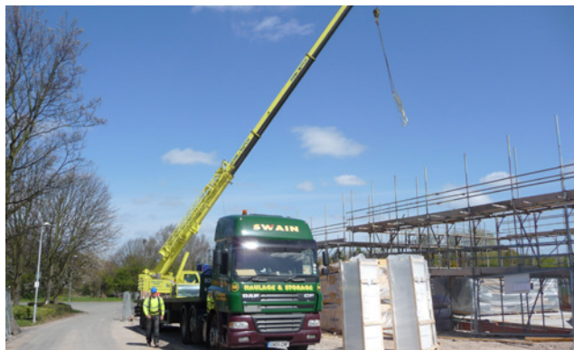
Figure 16 Closed panel timber frame units and air source heat pumps were unloaded onsite and craned into place
