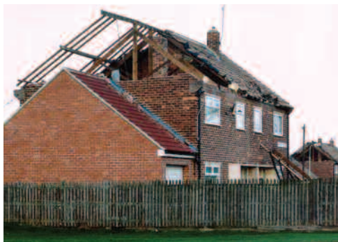
Figure 8 Wind damage to a roof.
