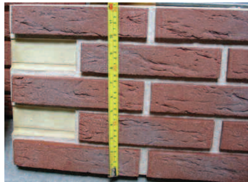
Figure 1 Cladding panel with non-standard brick slips.
