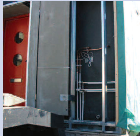
Figure 7 Accessible service riser.
