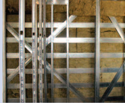
Figure 20 In addition to lateral bracing for structural stability this steel framed wall is also designed to keep out intruders.
