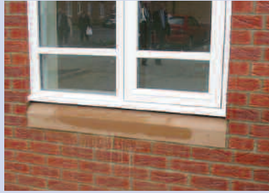
Figure 14 Sub-sills should project forward of the masonry to shed water away from the structure – flush sills as shown above should be avoided.
