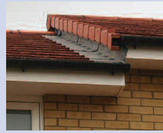
Figure 17 'Dry' verge and ridge systems can reduce the risk of wind damage in those locations.
