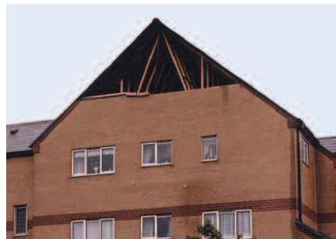
Figure 9 Wind damage to a gable wall.
