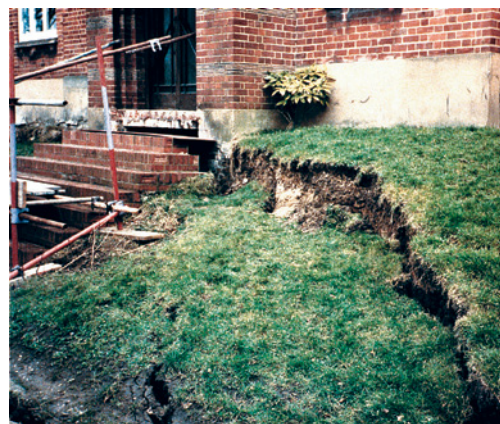
Figure 8 Damage due to landslip.
