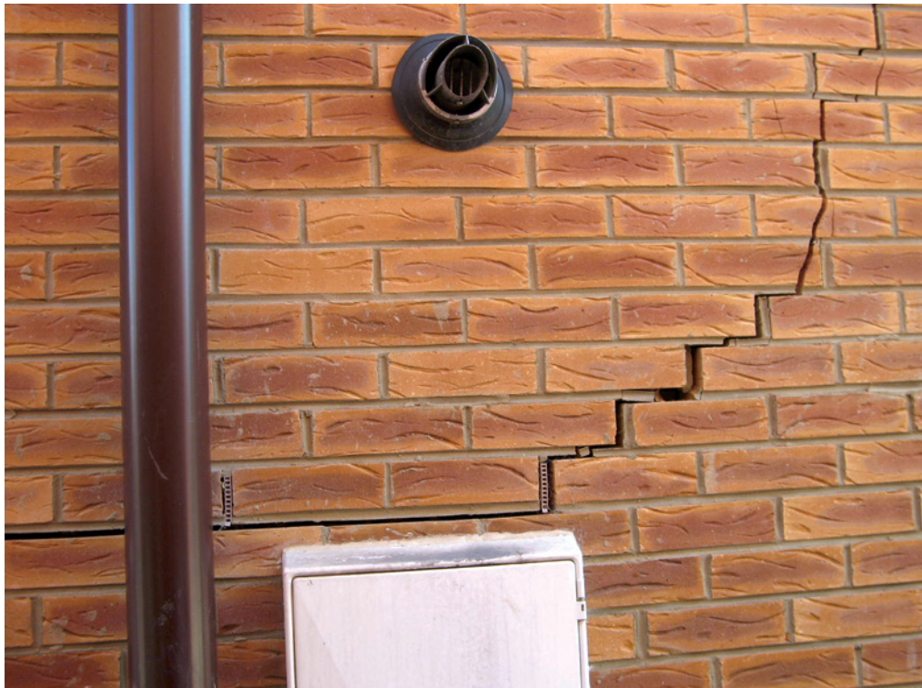
Figure 1 Example of structural damage of masonry caused by foundation movements.
