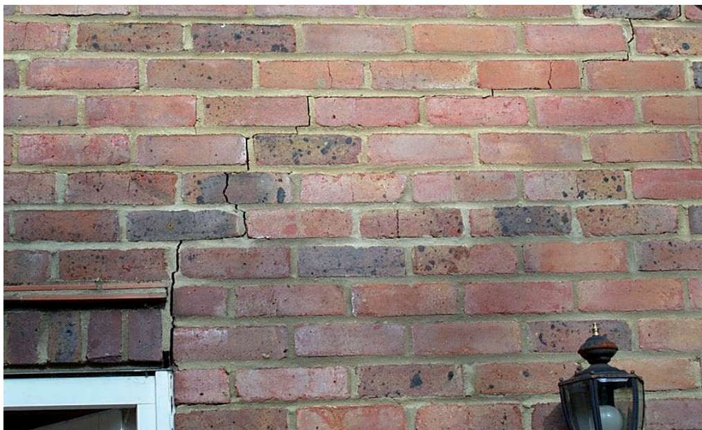
Figure 11 Damage to a property as a result of heaving clay soil beneath the ground beams where piled foundations have been used.
