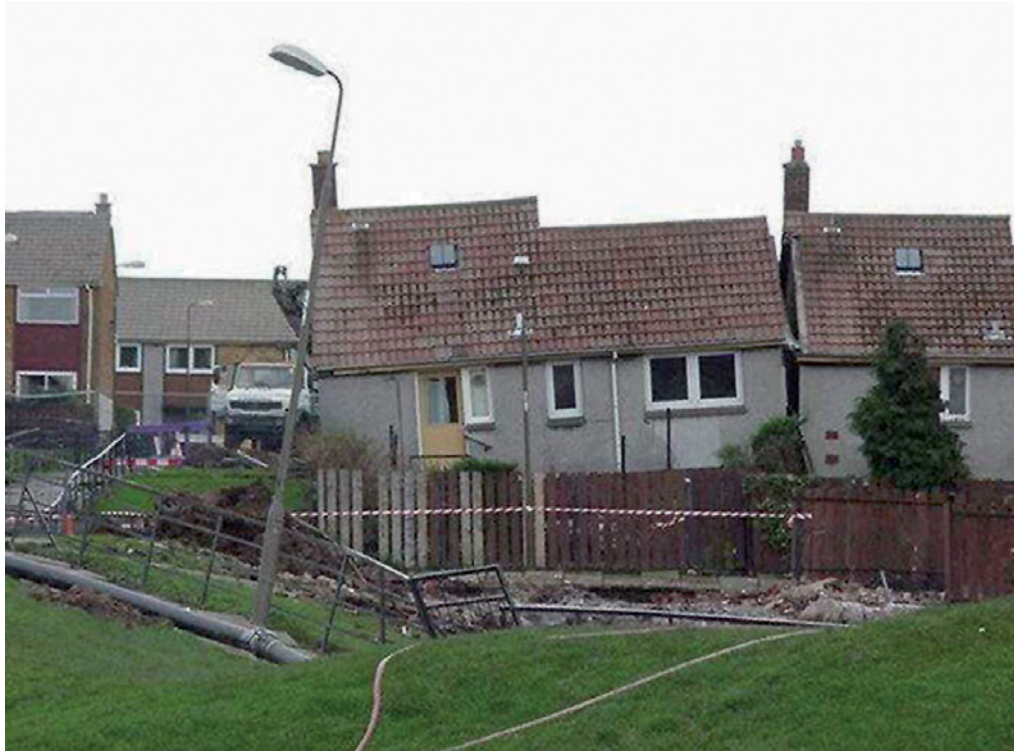
Figure 7 Subsidence associated with collapse of mining-related voids.
