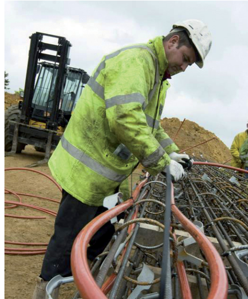
Figure K1 HDPE pipework being fitted to the reinforcement cage for a pile.
