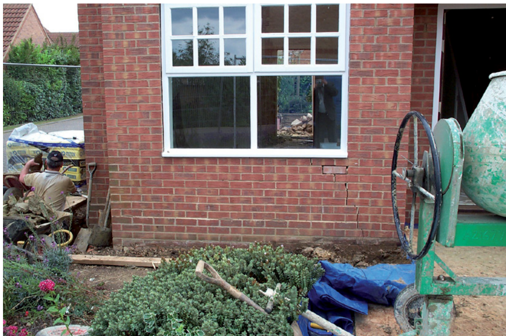
Figure 3 Example of damage, underpinning works are currently underway to prevent further movement occurring.
