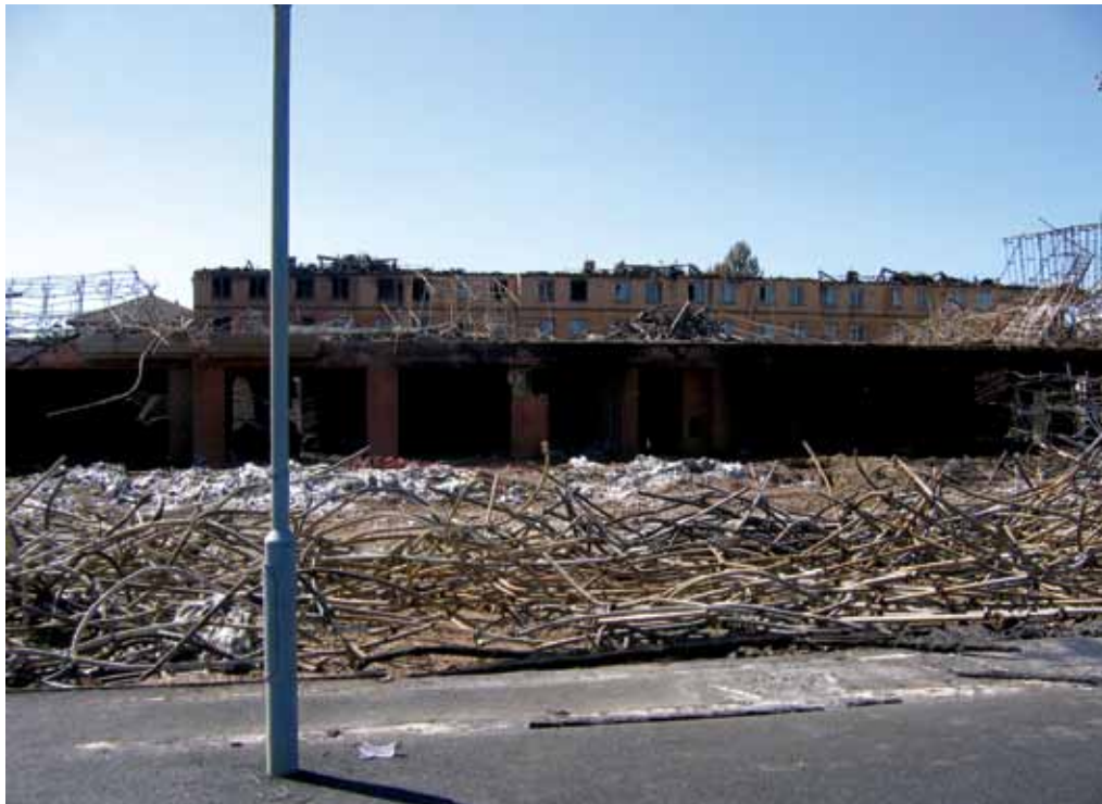
Figure 37 Extent of damage to roof structure of student accommodation opposite blocks B4 and B3
