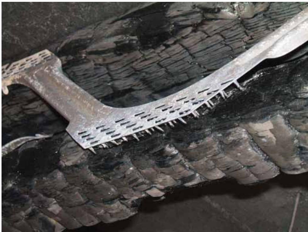
Figure 30 Loss of fixity between steel web elements and lower timber chord
