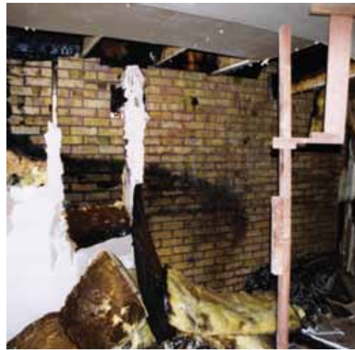
Figure 21 Loadbearing wall completely consumed by the cavity fire (3rd floor) of the TF2000 building
