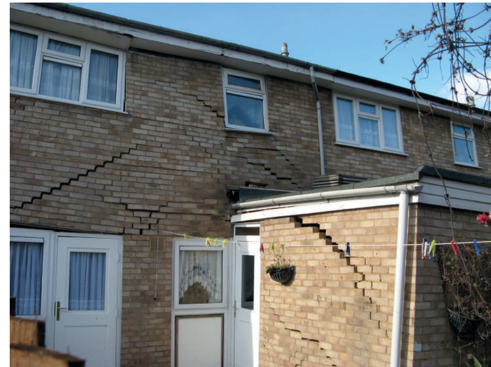
Image 5 Damage to housing caused by a solution feature or denehole (Source: RSK)
