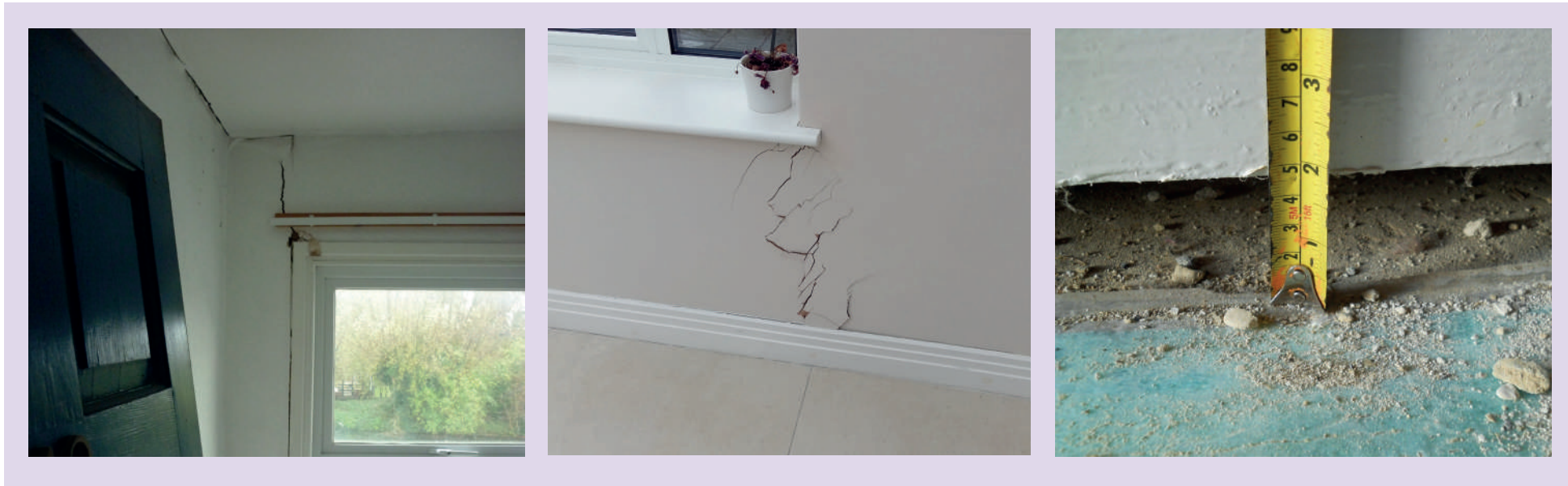
Image 3a-c: Examples of building damage caused by subsidence (Source: RSK)
