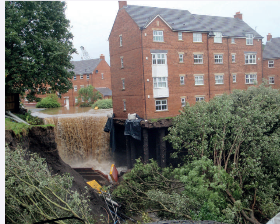
Image 4 Catastrophic damage caused by north-east floods, 2012 (Source: Tyne and Wear Fire Rescue Service)
