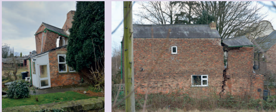
Image 6a-b: Sinkhole damage, Ripon, February 2014 (Source: BGS)
