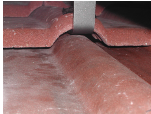
Figure 14 Hook fixing at top of tile profile increasing the tile gaps (not recommended).
