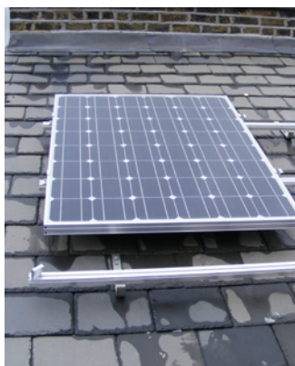
Figure 21 Bolt-through hook fixing on a slate roof (not recommended).
