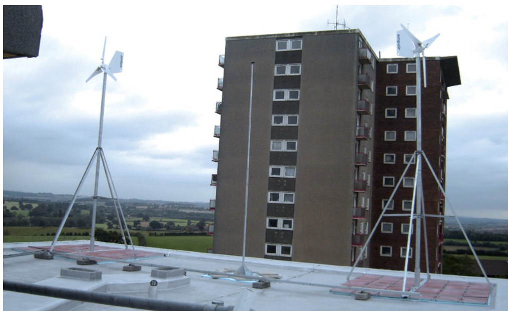
Figure 38 Microwind turbines installed on a flat roof.
