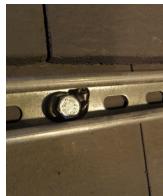
Figure 22 Example of a non-durable weather seal around a bolt-through fixing (should not be used).
