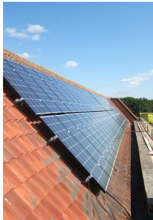
Figure 11 Above-roof PV system.
