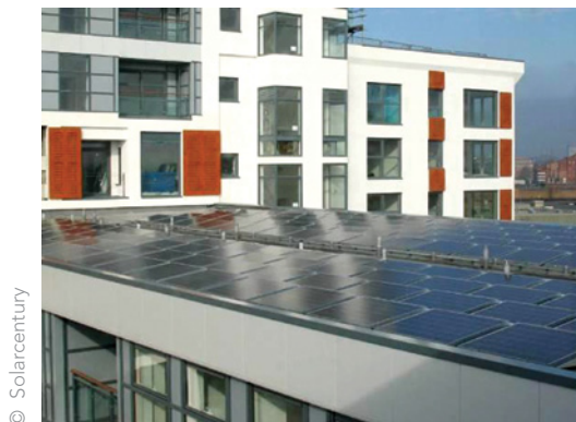
Figure 24 PV arrays mounted on a flat roof.
