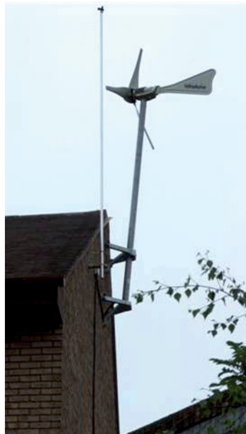
Figure 35 Failure of a microwind turbine fixing bracket into a masonry wall.
