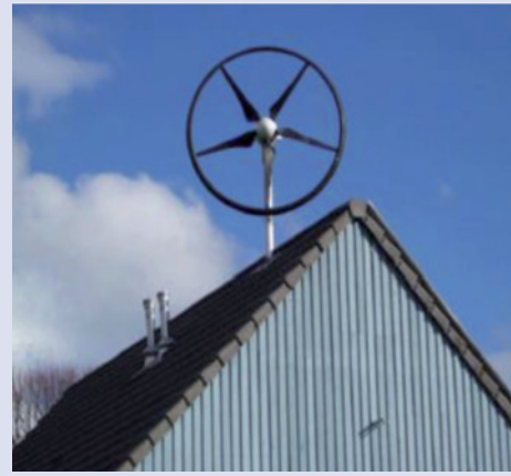
Figure 37 Wind turbine mounted through the roof.
