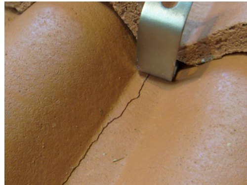
Figure 15 Tile damage caused because the tile was not notched around the hook.
