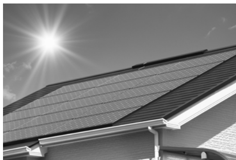
PV panels – often several flat panels per house
