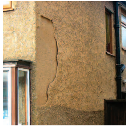
Figure 8 Poorly specified render with detaching final coat.
