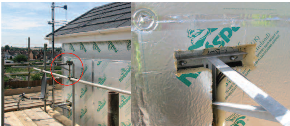
Figure 4 The bracket for aerials and satellite dishes has a lower brace that will encourage water to track towards the building.
