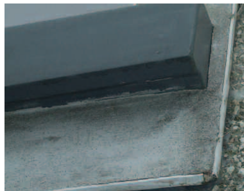
Figure 19 Gap around sill.
