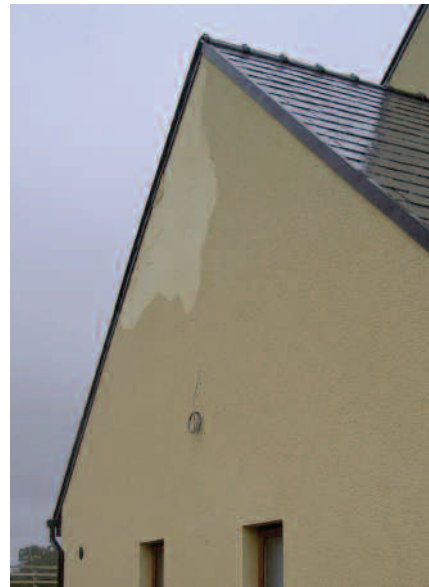
Figure 12 Polymer render failure.
