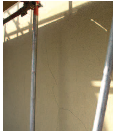
Figure 13 Cracking in newly applied polymer render.
