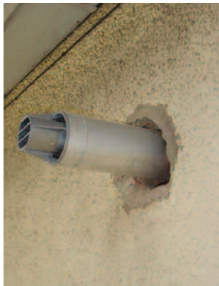
Figure 20 Extended boiler flue.
