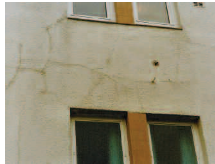
Figure 9 Cracking in render typical of a strong mix.
