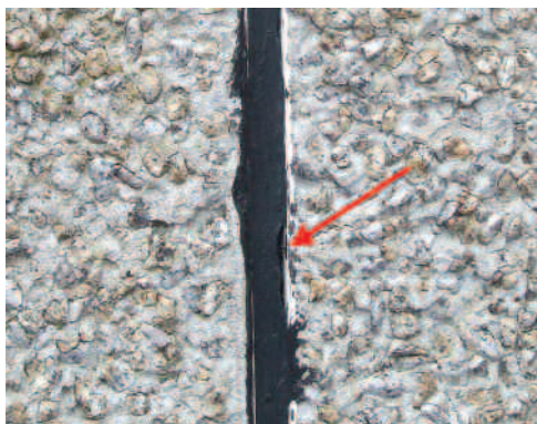
Figure 18 Movement joint with bond failure in mastic.
