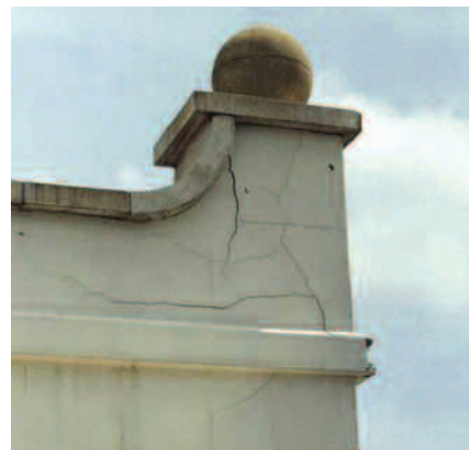
Figure 11 Example of sulfate attack on cement render on a parapet.
