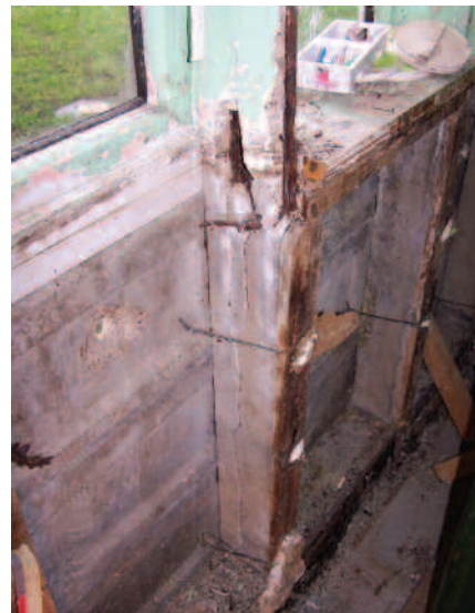
Figure 15 Cracking to PRC column in Airey house.
