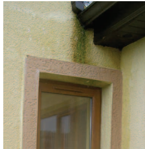
Figure 6 Water has penetrated behind the raised decorative feature.
