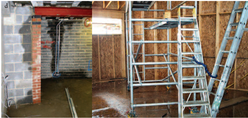
Figure 7d Structures becoming wet during construction.
