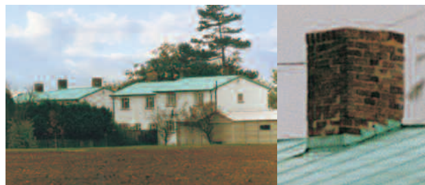
Figure 14 Copper-covered roofs on houses in open country. These roofs were laid in 1947 and have given excellent service.
