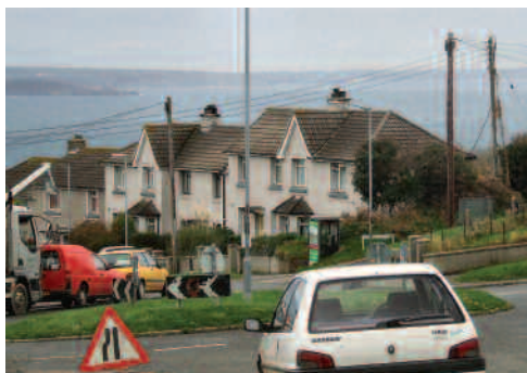
Figure 23 Good performance of 20-year-old render over external insulation.
