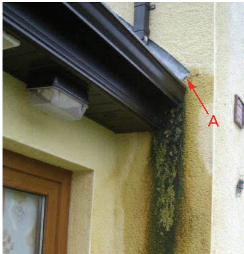
Figure 5 Poor detailing at junction.
