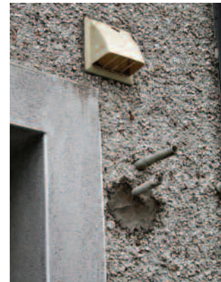
Figure 22 Various service penetrations.
