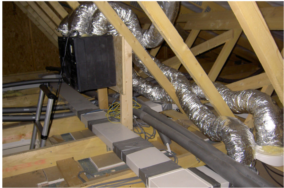
Figure 2 A complex arrangement of ductwork connecting to a mechanical ventilation and heat recovery unit
