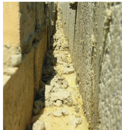
Figure 1 Poorly installed cavity wall insulation
