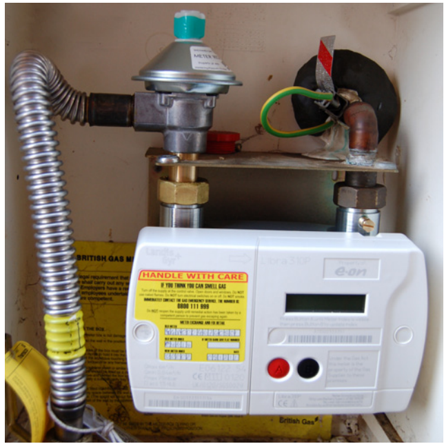
Figure 5 Smart gas meter
