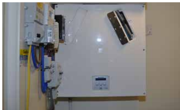
Figure 13 Ventilation filters that require cleaning and periodic renewal by occupiers
