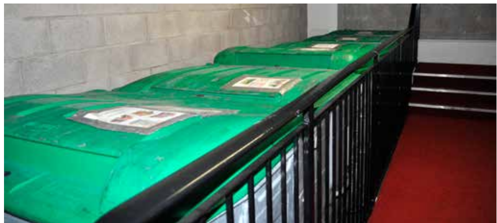
Figure 25 Challenges for refuse disposal with steps down to the platform and large heavy side-opening lids to bins
