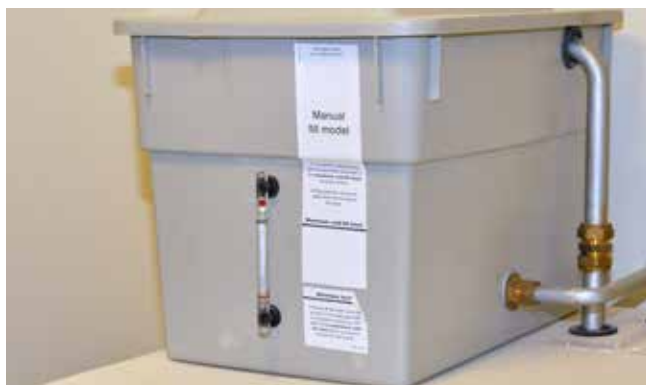
Figure 12 Hot water primary system header tank that requires manual top-up with water as necessary
