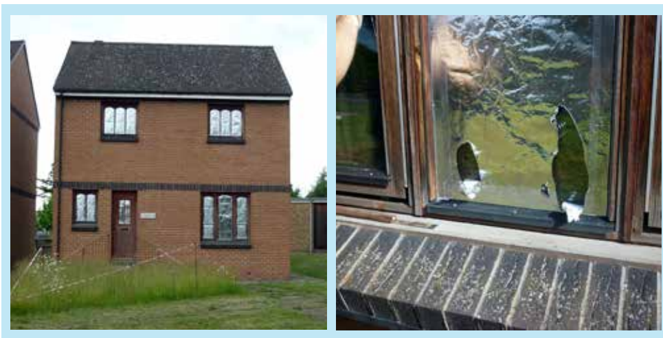
Figure 24 House B with aluminium foil attached directly to the glass on the outside of the window
