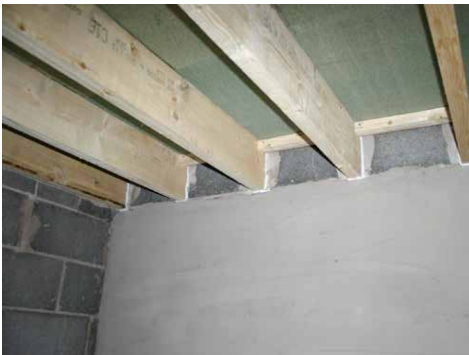
Figure 11 Minimising noise transmission (AD E E1) between new homes. Separating wall and floor joist detailing to minimise sound transmission
