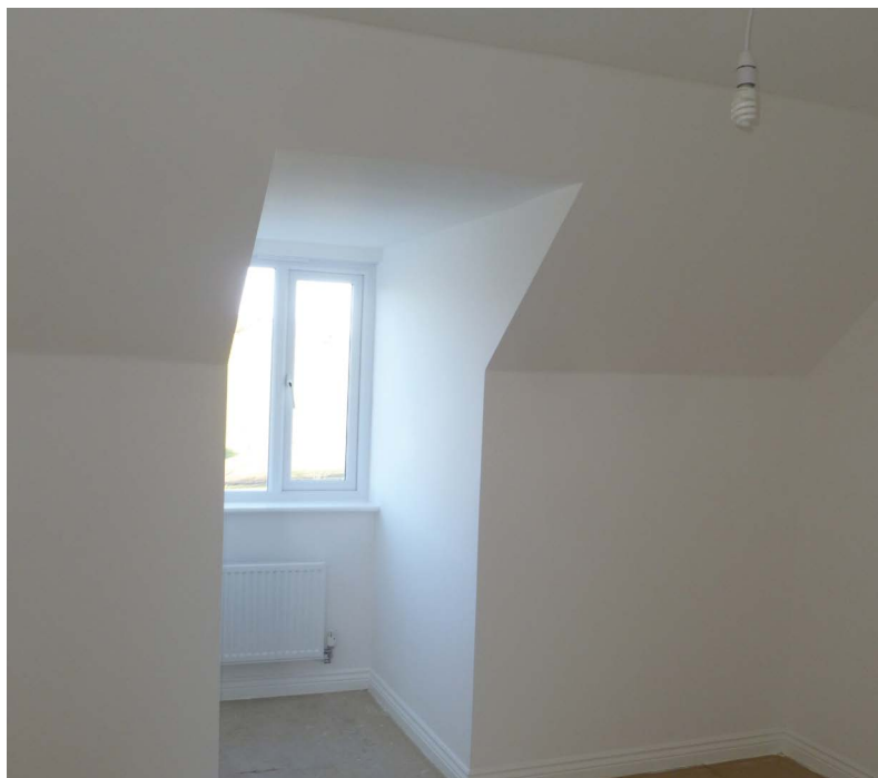
Thermographic image 19: Good construction
