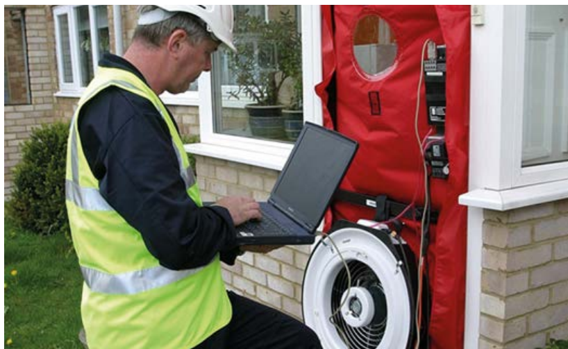
An air tightness test being carried out using a blower door kit
