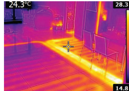
Figure 18 Surface temperatures across the floor of the same room not uniform due to incorrect commissioning
