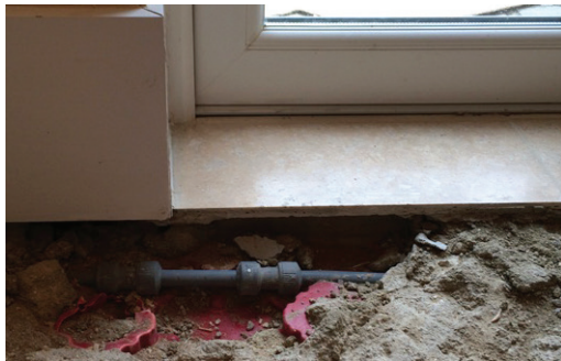
Figure 11 Pipework joint embedded in screed – this will be difficult to reach for repairs in the event of a leak developing
