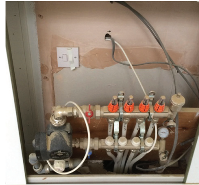
Figure 12 Manifold installation not secured onto wall – this could cause damage to both the wall and the components of the assembly
