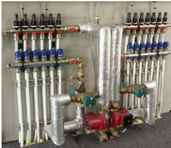
Figure 7 Well-insulated primary pipework at connection with manifolds
