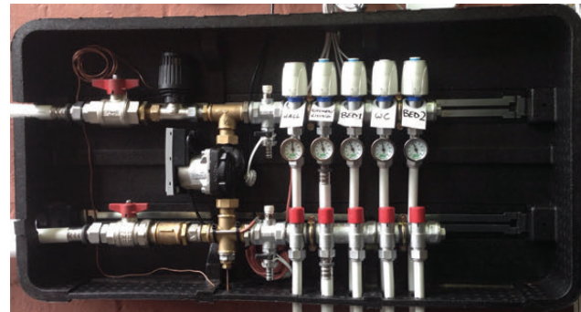
Figure 13 Manifold installed in a dedicated casing fixed to the wall. This can also have a cover made of insulating material to limit heat losses. These should be designed by the system manufacturer to prevent any risk of overheating of components
