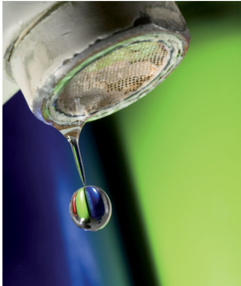
Figure 11 Build-up of limescale on an aerating tap outlet.
