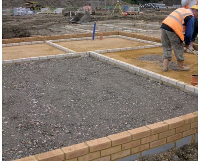
Figure 3 Hardcore in place and being blinded with sand (© Bellway Homes East Midlands)
