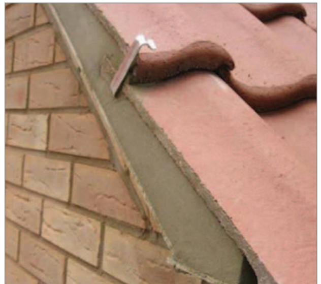
Figure 7: Ensure clips are correctly installed - unlike this one
