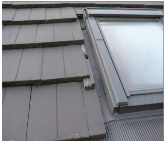
Figure 5: Failure of small sections of cut tiles
